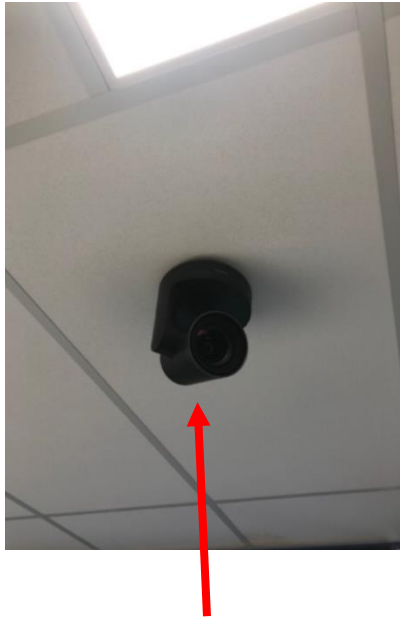
Ceiling Mounted Camera in Rooms G02 and G04
