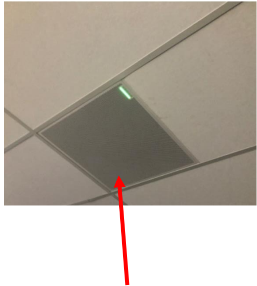
Ceiling Mounted Shure Microphone array to use in Teams Town Hall setups – located in all Rooms; G01 through to G04
